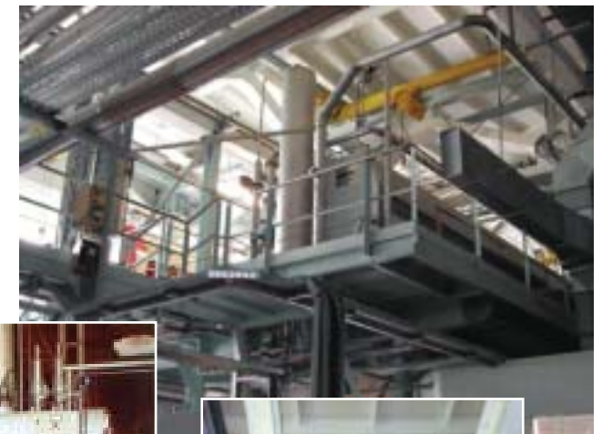
Meura 2001 mash filters : general view
